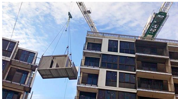
Figure 2: The construction of a residential apartment using the MiC concept. (Image provided by and reproduced from [15])
