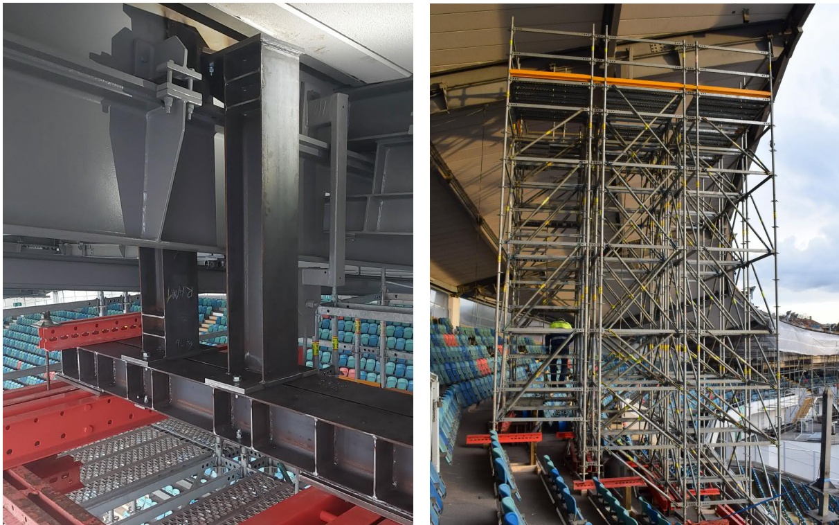
Figure 5: The roof prop adaptor (unpainted) and transfer beams (red) temporarily supports the roof primary beam (gray), exerting a load of 720 kN on the scaffolding tower.
