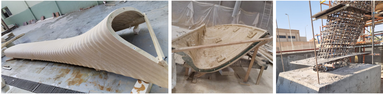
Figure 12: Mold used for formwork production (left), UHPC lost formwork (middle), trial mockup showing in-situ steel reinforcement awaiting placement of lost formwork and casting.
