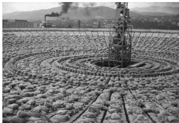
Figure 6: The process of prestressing the inverted dome of the Hall of Sports in Nis (UB-FA Archives)
