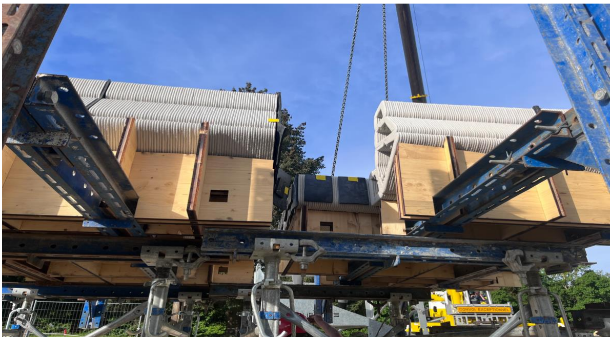
Figure 5: Referencing and preassembly of the building groups on pre-installed off-the-shelf adjustable scaffolding towers, (c) Serban Bodea
