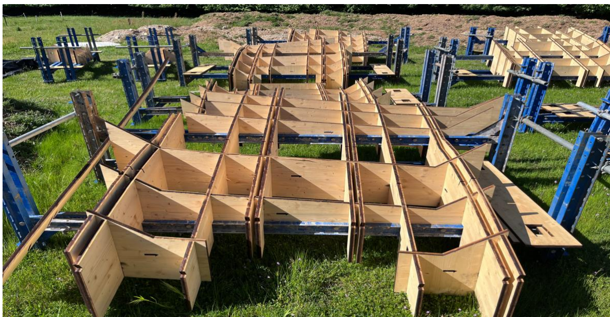
Figure 3: Preassembled falsework cassettes, including bespoke, laser-cut CLT elements on off-the-shelf formwork system components; (c) Serban Bodea
