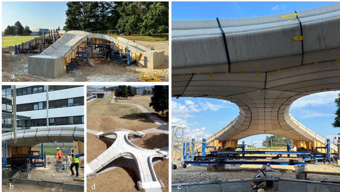
Figure 7: Phoenix assembly and decentering. a. Building Groups completely assembled on falsework system; b. Decentering process, partial removal of falsework under central section of the main arch, (c) Alessandro Dell'Endice; c. Decentering process, intrados view of the main bridge-arch with falsework nearly entirely removed, (c) Alessandro Dell'Endice; d. Overview of the structure with the falsework system entirely removed, (c) Cecilia Vuillermoz
