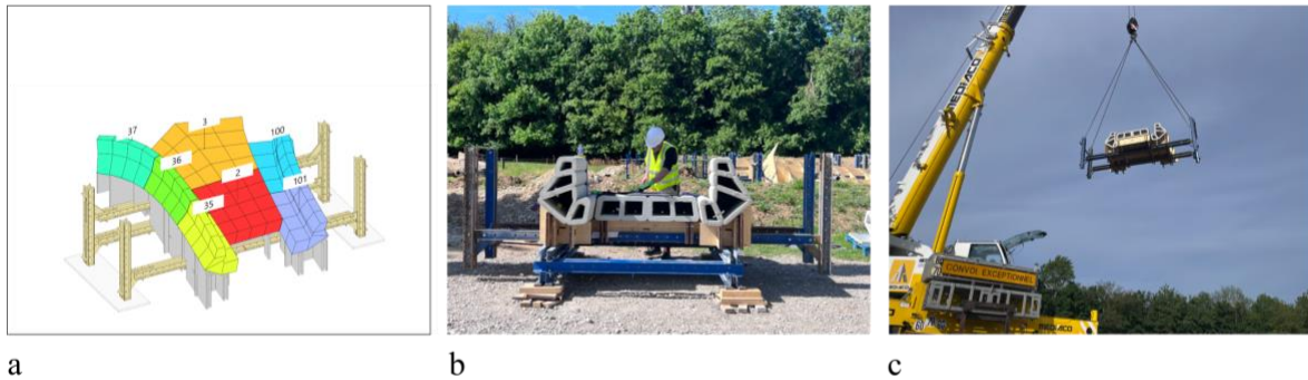
Figure 4: Preassembly process. a. Building Group 3D model, (c) Vasilis Aloutsanidis; b. Building Group assembled, (c) Serban Bodea; c. Building Group manipulation by construction crane, (c) Serban Bodea
