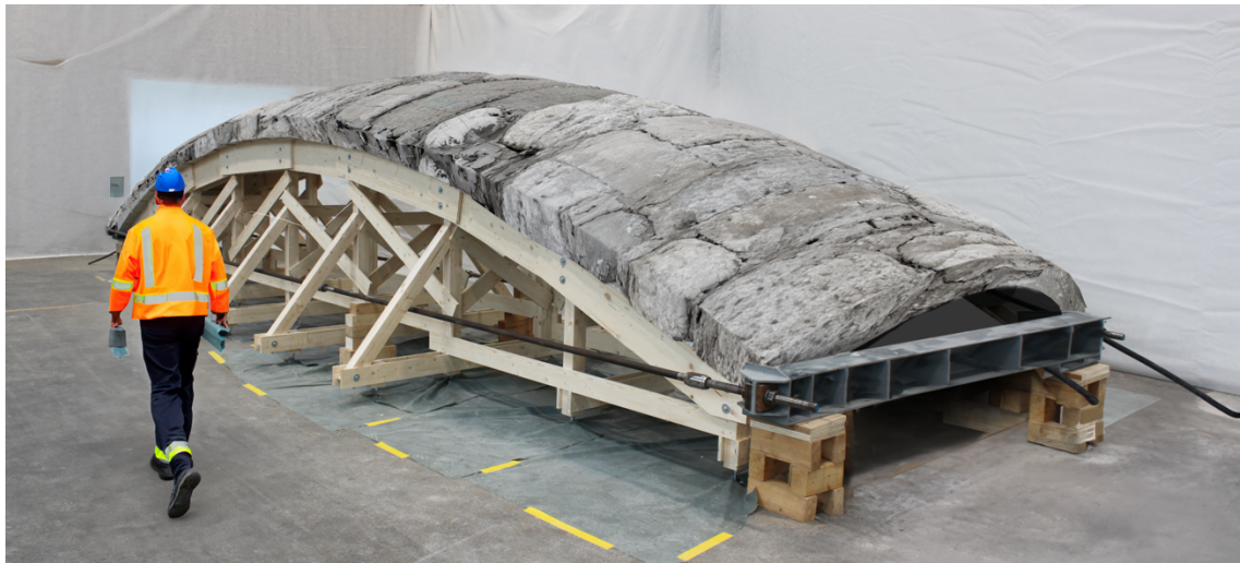
Figure 6: Collage by Grangeot of the prefabricated construction of an unreinforced masonry vault made of large flat demolition concrete rubble. The collage is used as an experimentation tool to plan constructive solutions.
