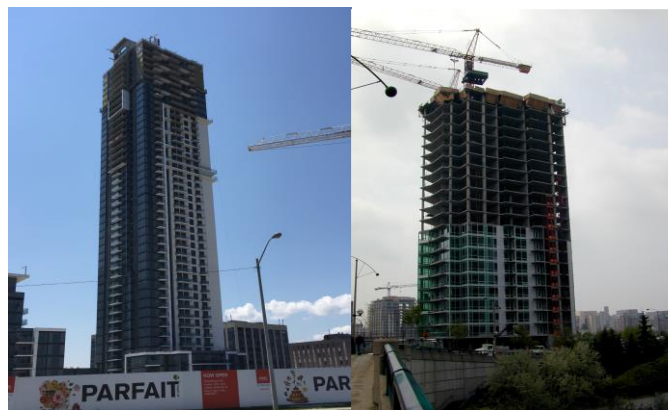
Figure 4: Two typical high-rise multi-unit residential buildings constructed using structural system B. Façades are a combination of Window Wall with precast concrete panels.
