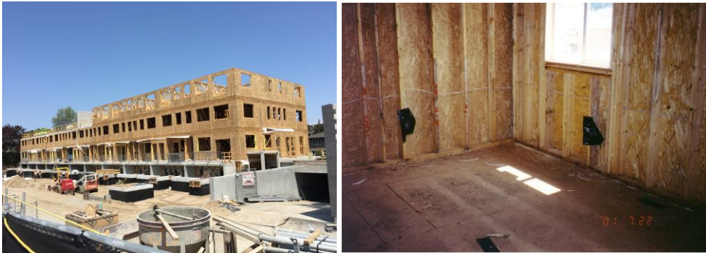
Figure 3: System A - typical row housing structure constructed using wood framing with an underground reinforced concrete basement/garage.
