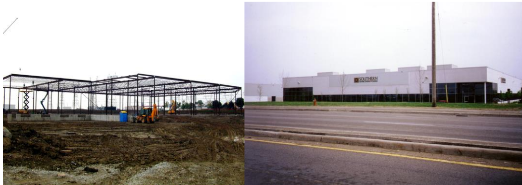
Figure 5: Typical building structure being constructed using System C and a finished building.
