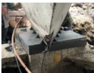
Figure 10: Steel plate to strengthen the connection between the footing concrete cap and the shell's groin.
