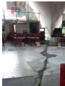
Figure 6: Crack on the earth that damaged the shell.
