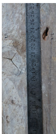
Figure 6: measurement of the wood defects
