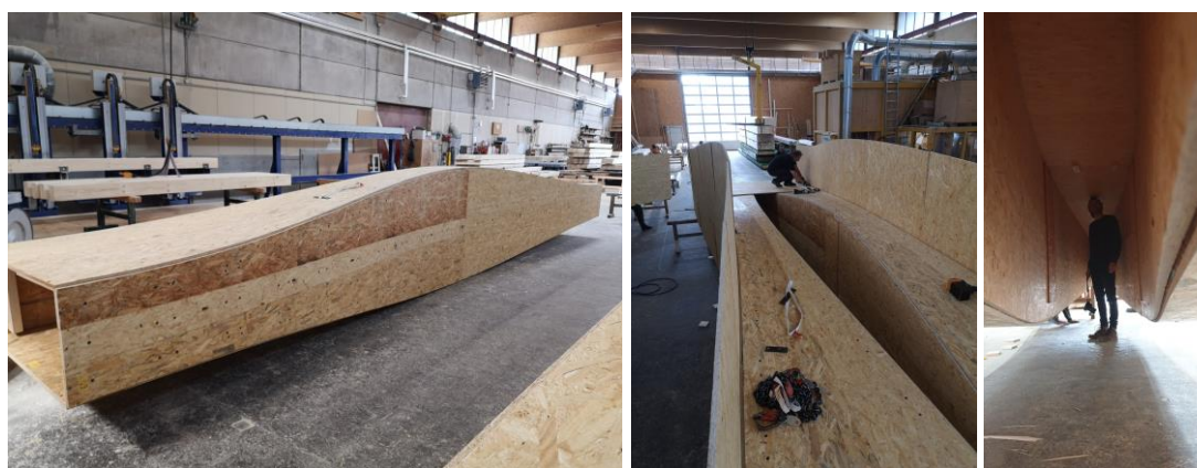
Figure 11: One final beam element (left) and the bridge consisting of two beams during construction (right)
