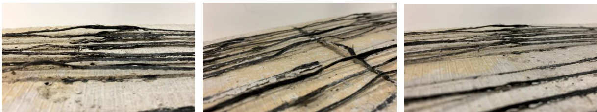
Figure 8: Carbon fiber detachment from concrete during formwork removal
