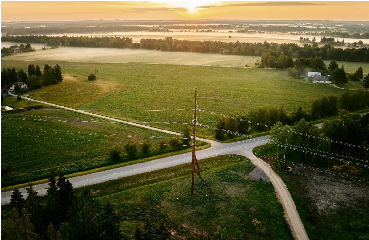
Figure 7: Bog Crane , a prototype for a carrying pylon that is carrying 3x 330kV phases, 3x 110kV phases and 2x earth wires [Image: Tõnu Tunnel]
