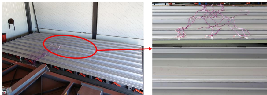
Figure 10: Roof panel seam disengagement
