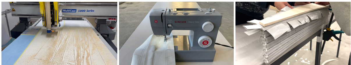
Fig. 6: Prefabrication of the CCU formwork: (a) cutting of the plywood plates, (b) sewing of the textile strips, and (c) assembly of the CCU system
