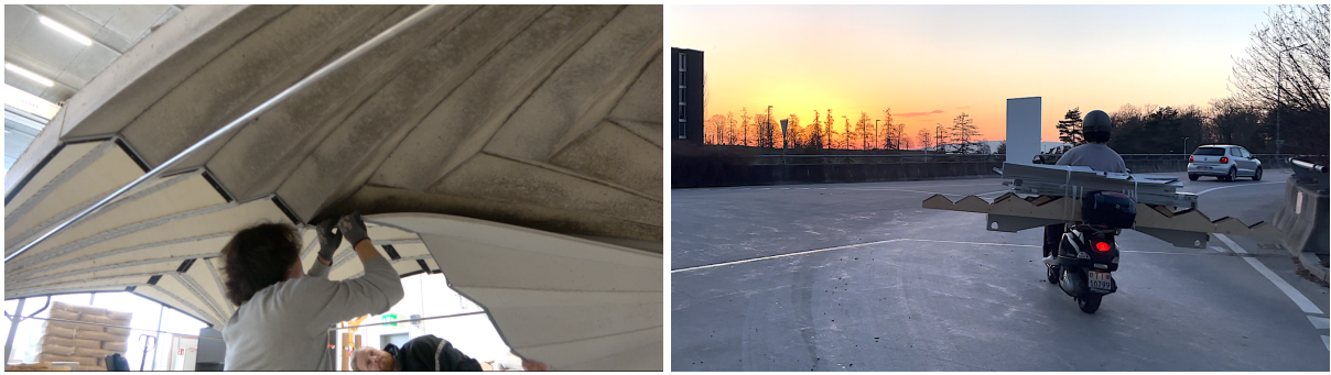
Fig. 9: (a) Decentring of the CCU quarters, and (b) transport of the formwork on a Vespa for reuse
