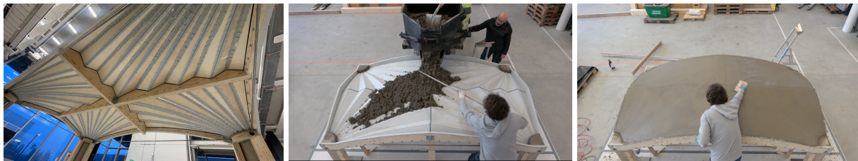
Fig. 8: Concrete casting: (a) underside of formwork, (b) filling of the triangular-shaped ribs, and (c) manual shaping of the shell's extrados with masonry trowels
