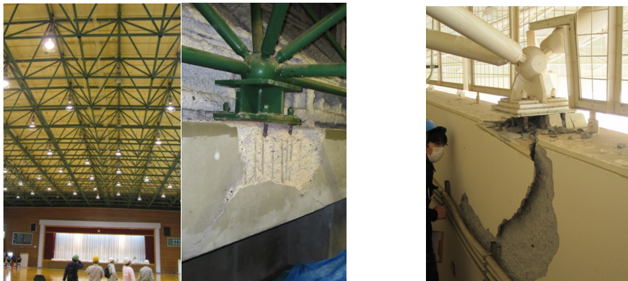
Figure 2: Damage of roof bearings supported by cantilevered RC wall [2]
